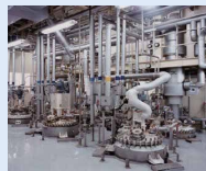
Facility for producing phospholipids for pharmaceuticals
